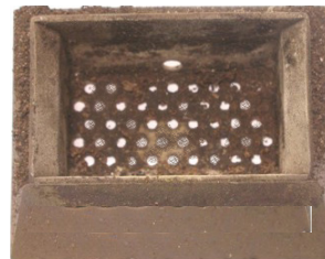
Fire pot needing cleaning with the holes blocked by ashes
